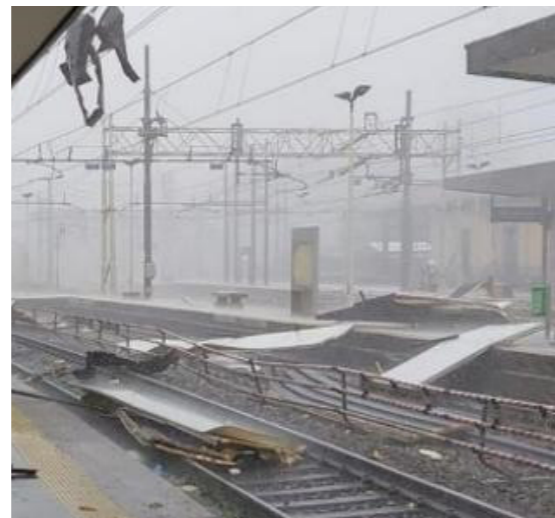
Broken canopies in Monza station
