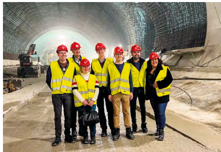
TPM Working Group visiting the Terzo Valico construction site on the occasion of its meeting in Genoa.
