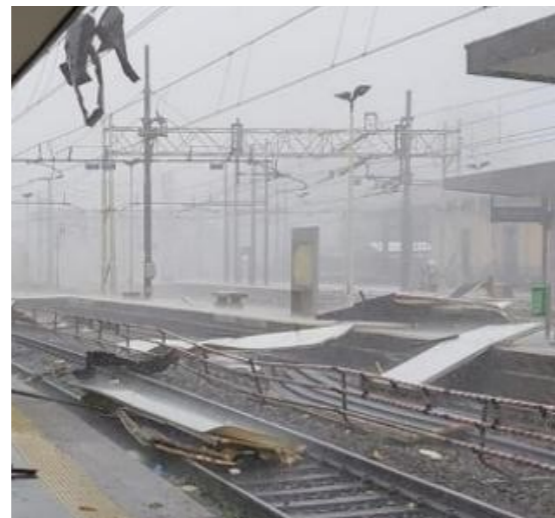
Broken canopies in Monza station
