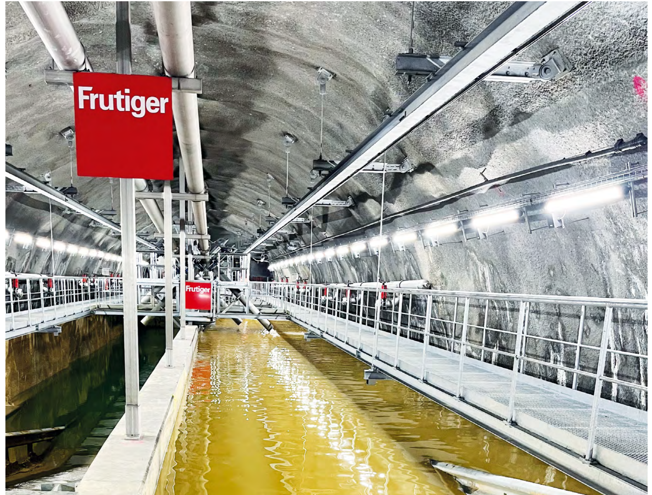
Cavern with sediment basins to collect and filter sand out of the karst-breakthrough in the Lötschberg Base Tunnel.
