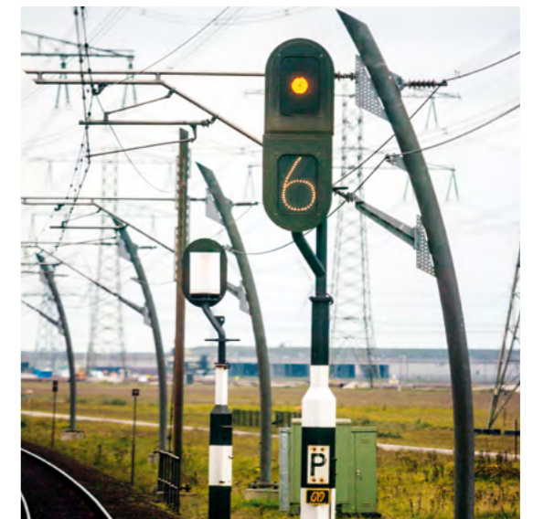
Dutch light signal along the Corridor.
